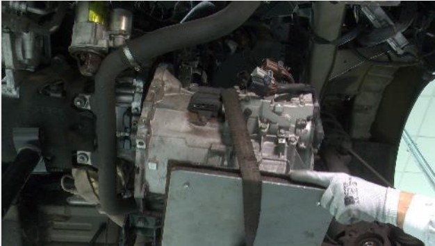
STEP 4 - Reassembly gearbox using the hydraulic lift table smoothly until DDC and flywheel are completely fitted
